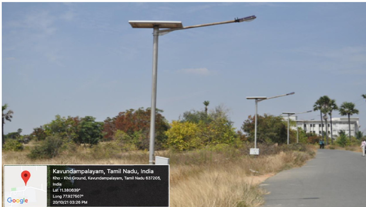
Four 10W LED Solar Street Lights in Sengunthar Engineering College Campus
